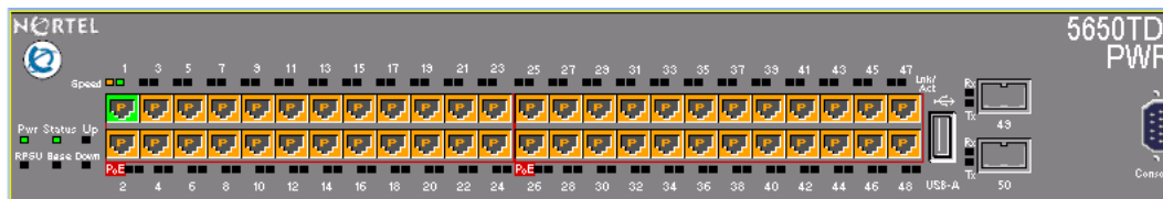
Figure 26 Nortel Ethernet Routing Switch 5520-48T-PWR
